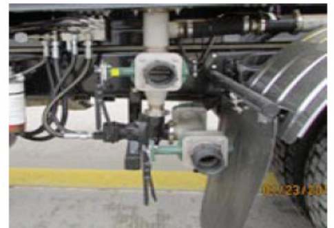
3" X 2 1/2" Product Pump Stainless steel Plumbing
